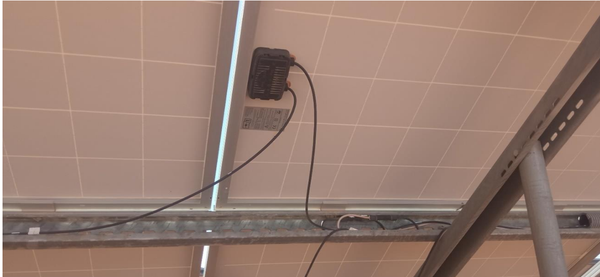
Figure II.3. Les câbles des raccordements
