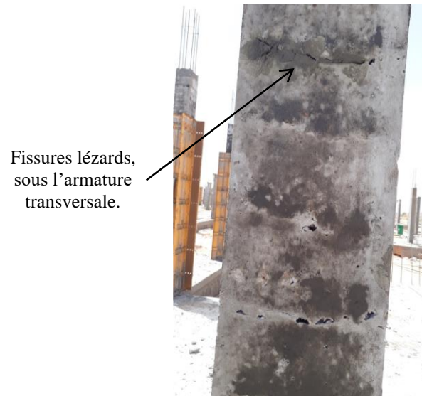
Photo 2.4. Fissures apparentes lézards.
