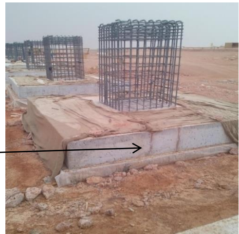
Photo 2.58. Fissures aux semelles.
