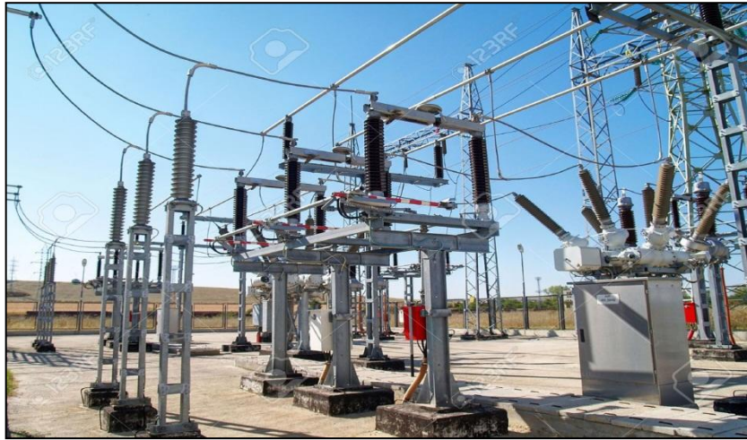
Figure 2.6: A High Voltage Electrical Substation [25]
