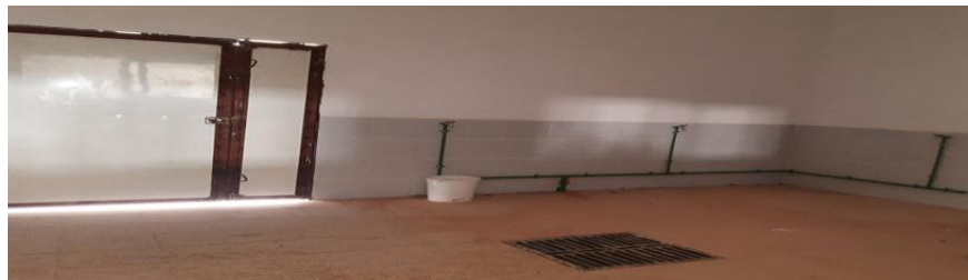
Figure 22; salle de lavage
