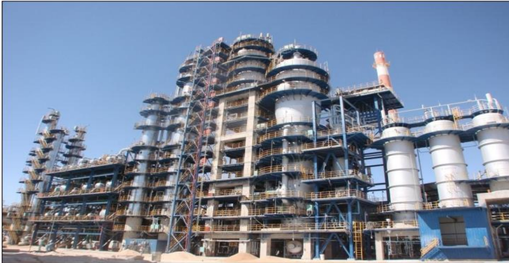
Figure I.33 Catalytic cracking unit
