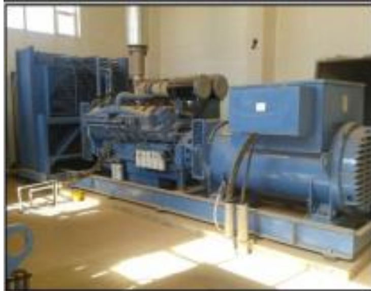
Figure I.58 Turbo diesel generator
