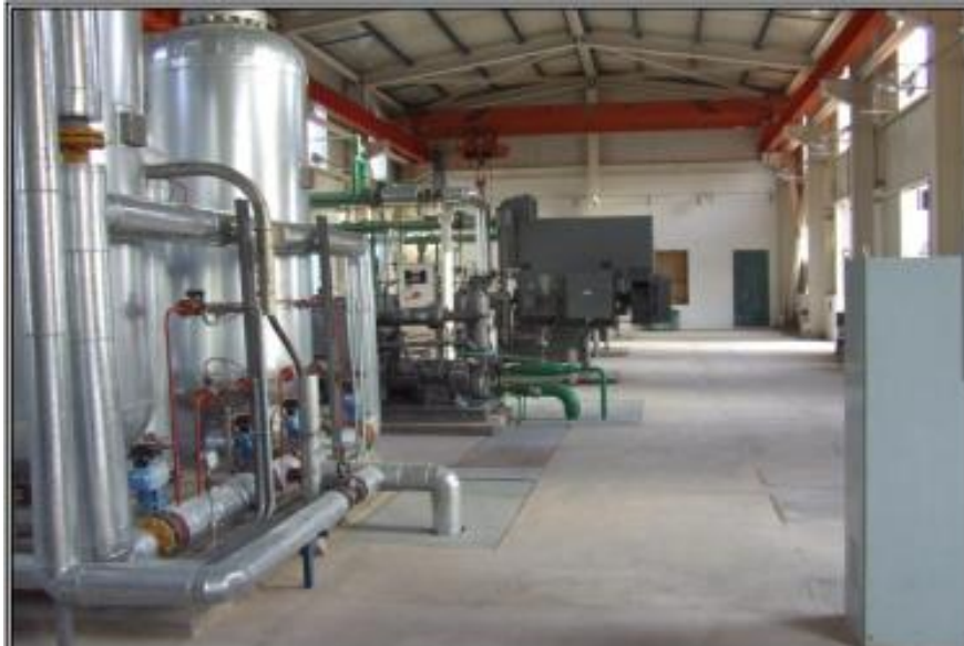
Figure I.69 Compressed air unit
