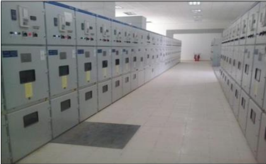
Figure I.64 Electrical Network Control Room
