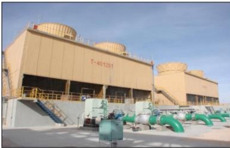
Figure I.72 Water cooling tower
