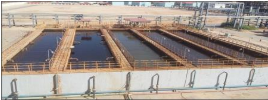
Figure I.43 Wastewater treatment tank
