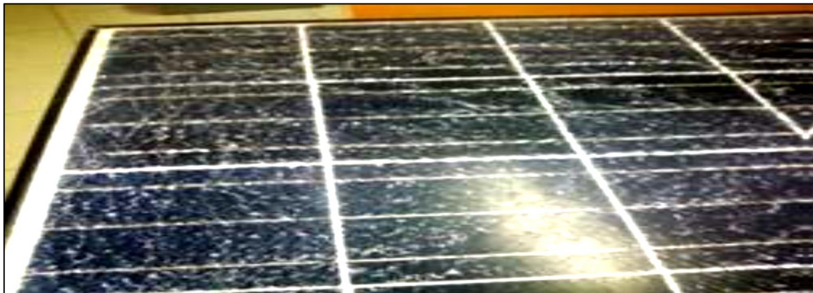
Figure II.23: Photovoltaic module with broken glass
