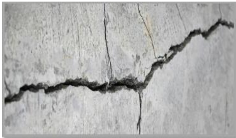
Figure II. 1: Fissuration du béton [2]
