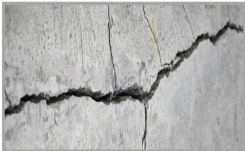
Figure I. 14: Fissuration du béton [1]
