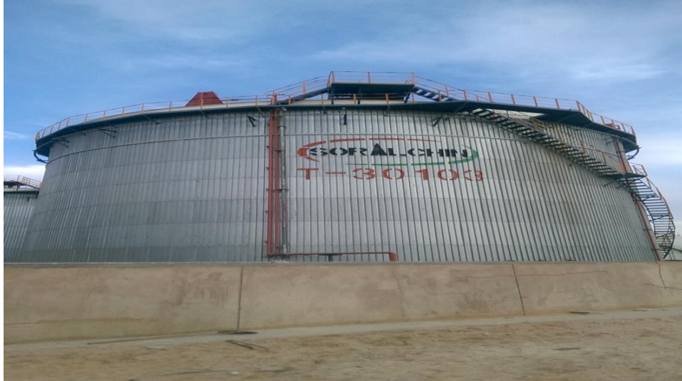
Figure I.11: Bac de stockage.
