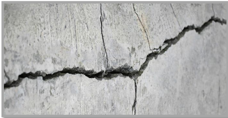
Figure 19: Fissuration du béton [43]
