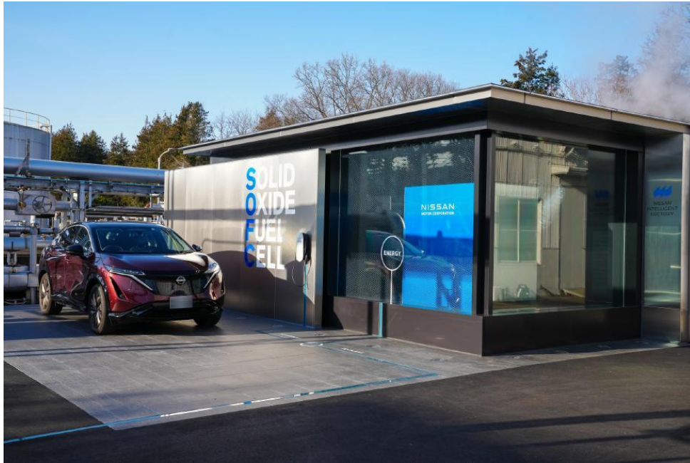
Figure 2.7: Stationary Power Generation:
