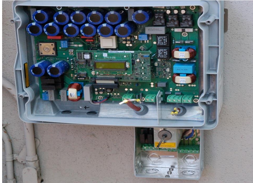
Figure 1.11: Inverters in a photovoltaic system
