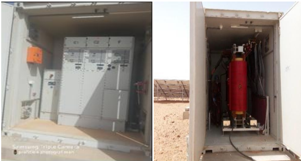
Figure II.20. Le transformateur SUNTEN ZBW10A-1250.
